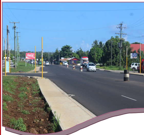
Extension of the four lane road Malifa to Vaitele, one of the Governments major infrastructural project implemented during the period
